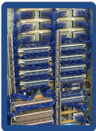
Railway Signalling Panel
