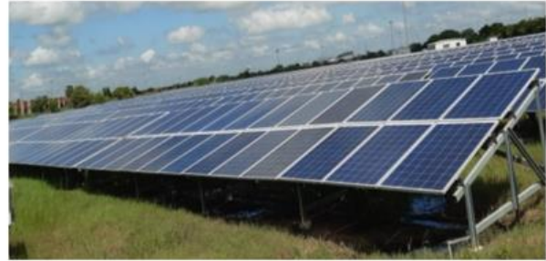
3 MW Solar Land Based Project at Modern Coach Factory, Raebareilly
