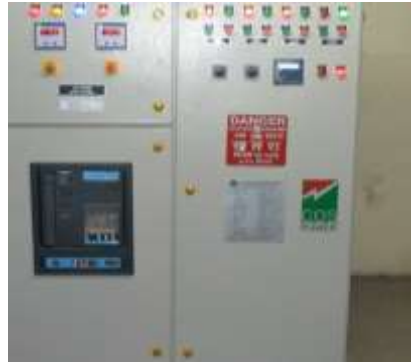
LT APFC (Automatic Power Factor Control) panels with contactor based switching
