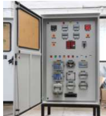
Control and Relay Panels
